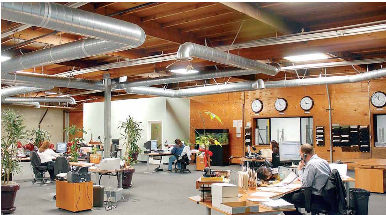
A-1 Cold Storage has no out-facing windows yet this office is daylit by Ciralight SunTrackers and all electric lights are off!
