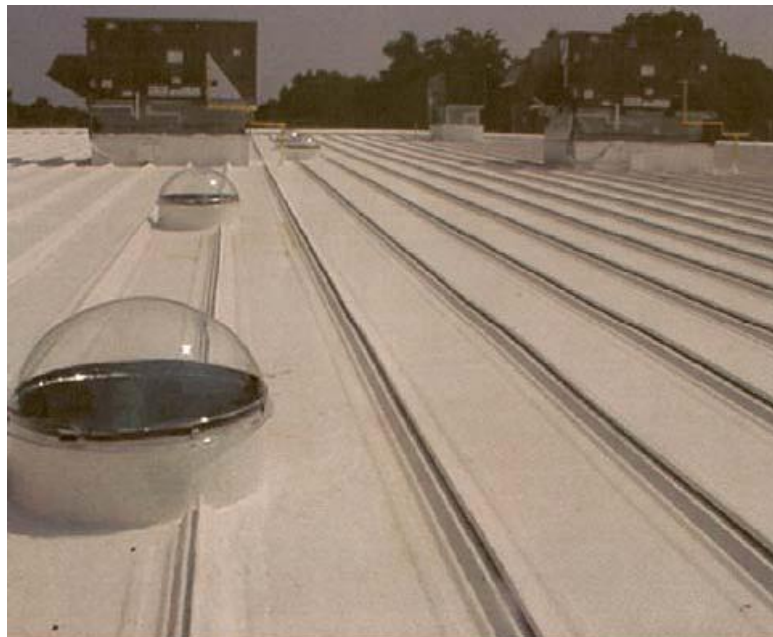
This installation is on a standing-seam metal roof.
