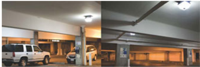
With bi-level lighting, energy is saved when the lights are dimmed and higher color temperature lighting provides for an improved visual environment.
