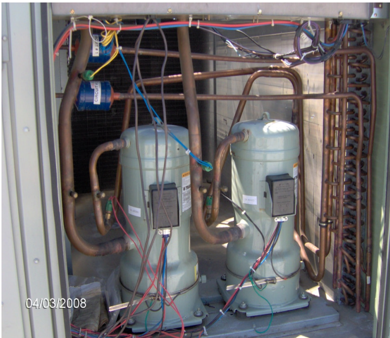
Original Compressors. compressors.
