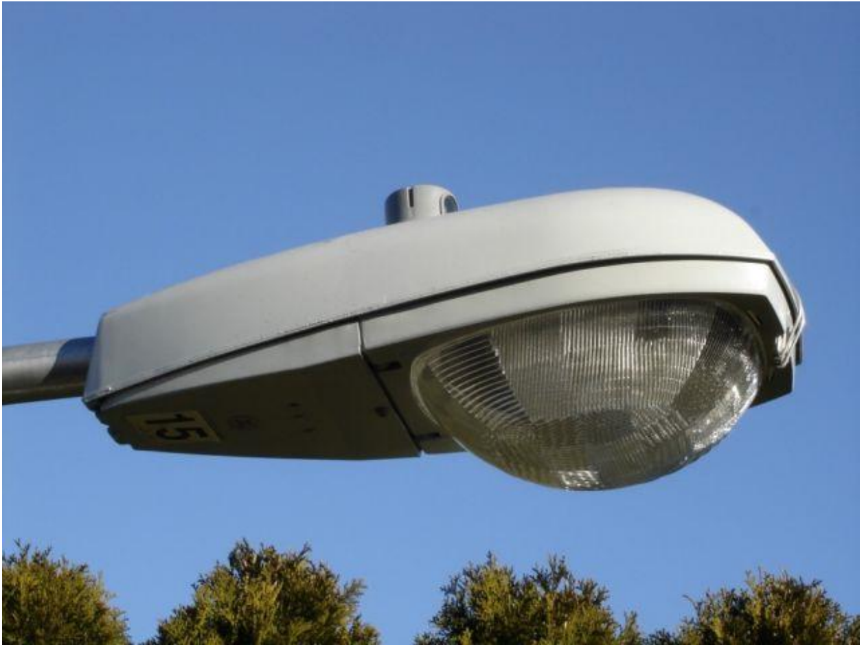
Parking Lot Pole Mounted Cobrahead Fixture
