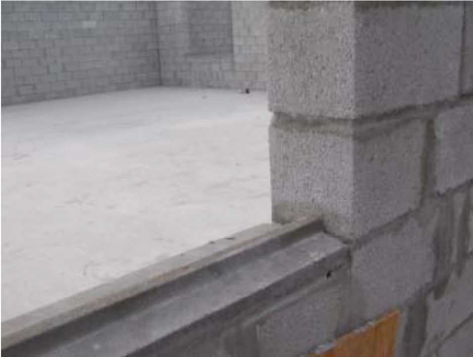
Photograph 28: Precast Sill That Channels Window Leakage Inward
