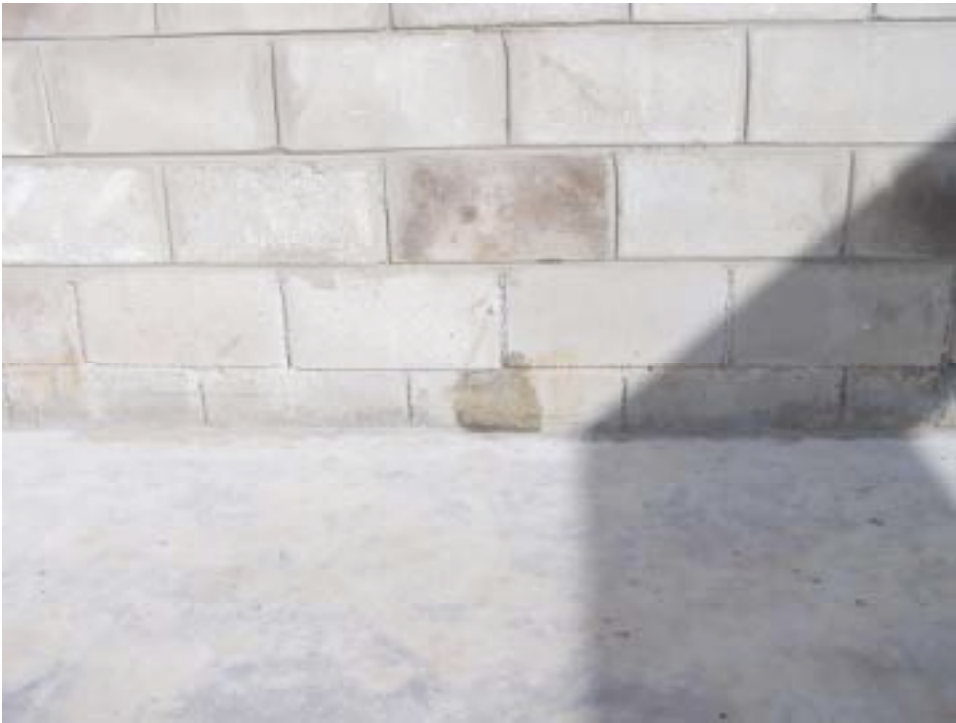
Photograph 55: Visual Indication of Water Entry At Base of Assembly
