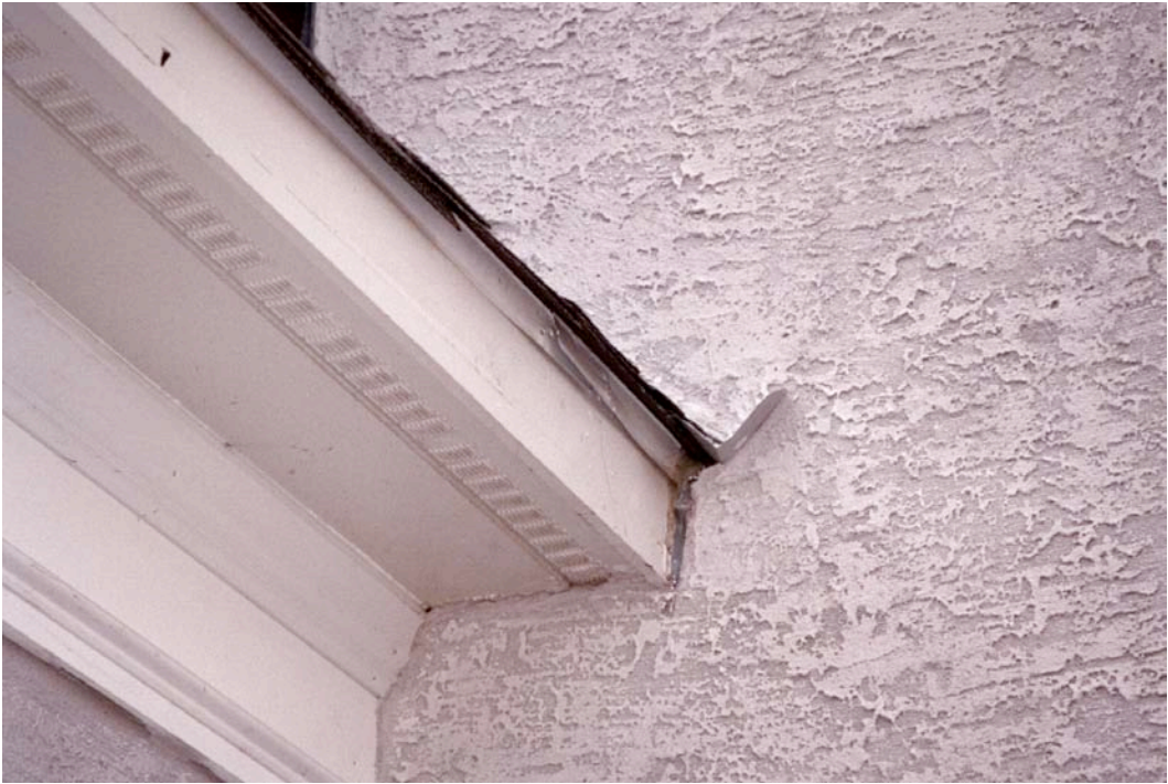
Photograph 39: Kick Out Flashing
