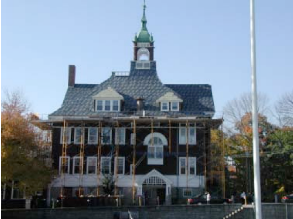
Photograph 74: Complex Roof Geometry – Direct Applied Self Adhering Membrane
